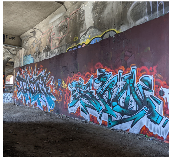
Graffiti in the historic Aqueduct level
